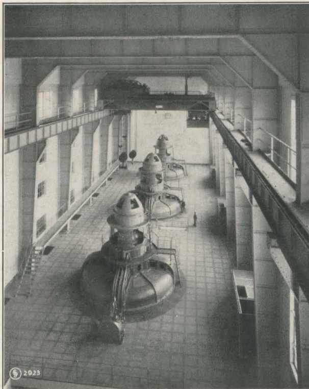
11. General view of the Generator Hall in the Power Station
