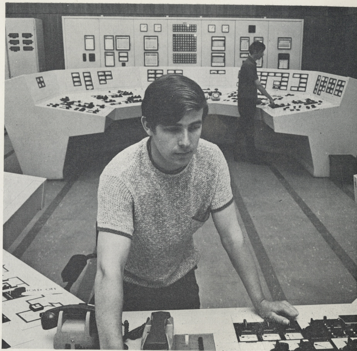
The control room at Tarbert. Power from the station is fed into the national grid. Electricity is generated at 10,000 volts and 'stepped up' to 110,000 volts at the transformers.
