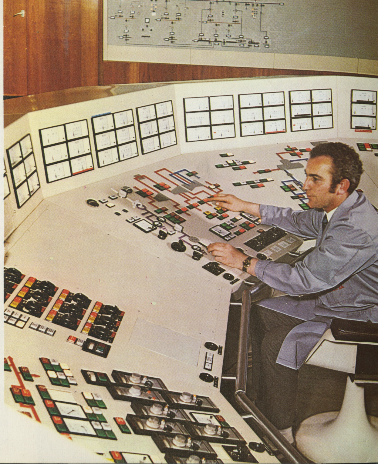
CENTRAL CONTROL ROOM
