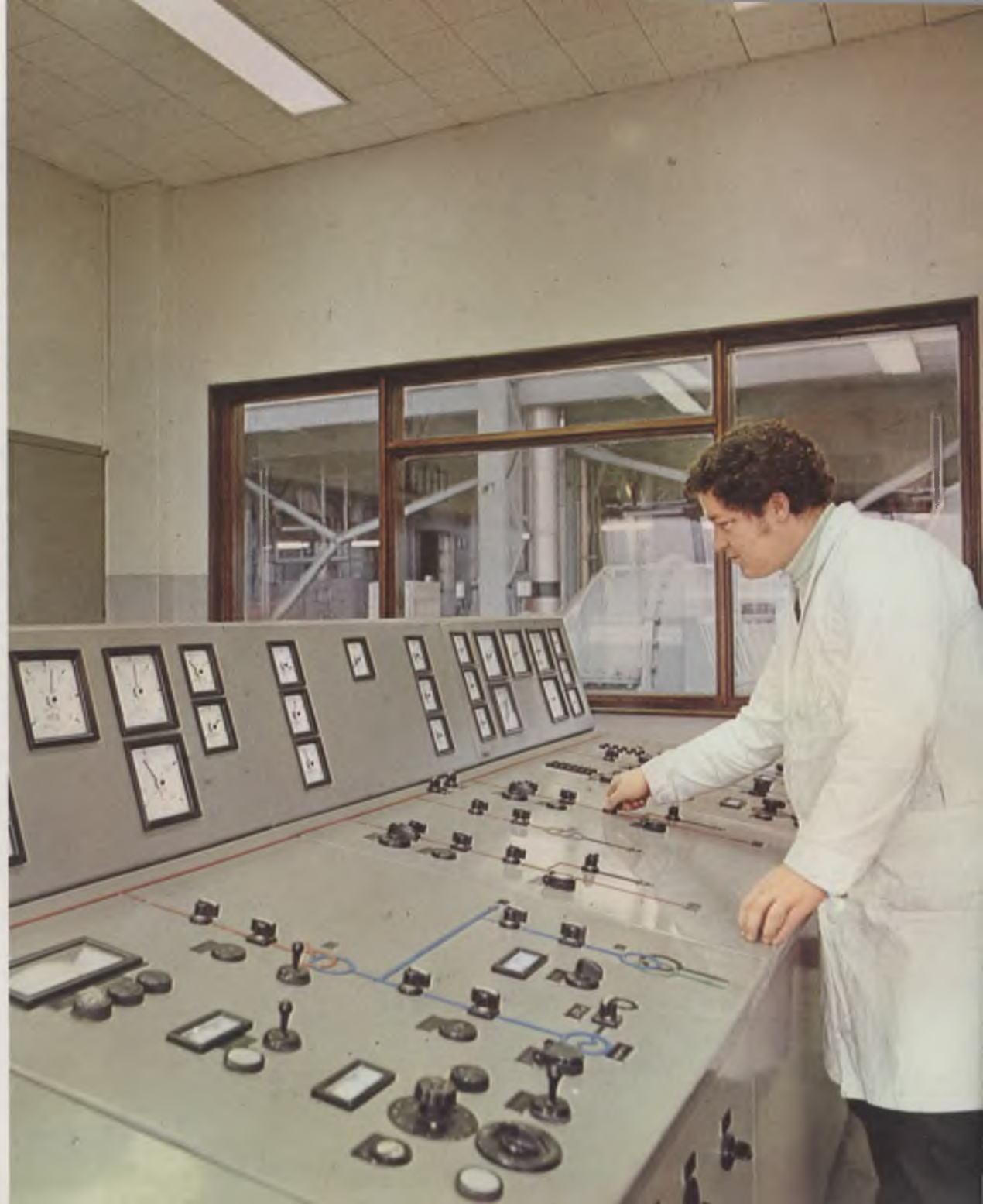
Electrical Control Room
