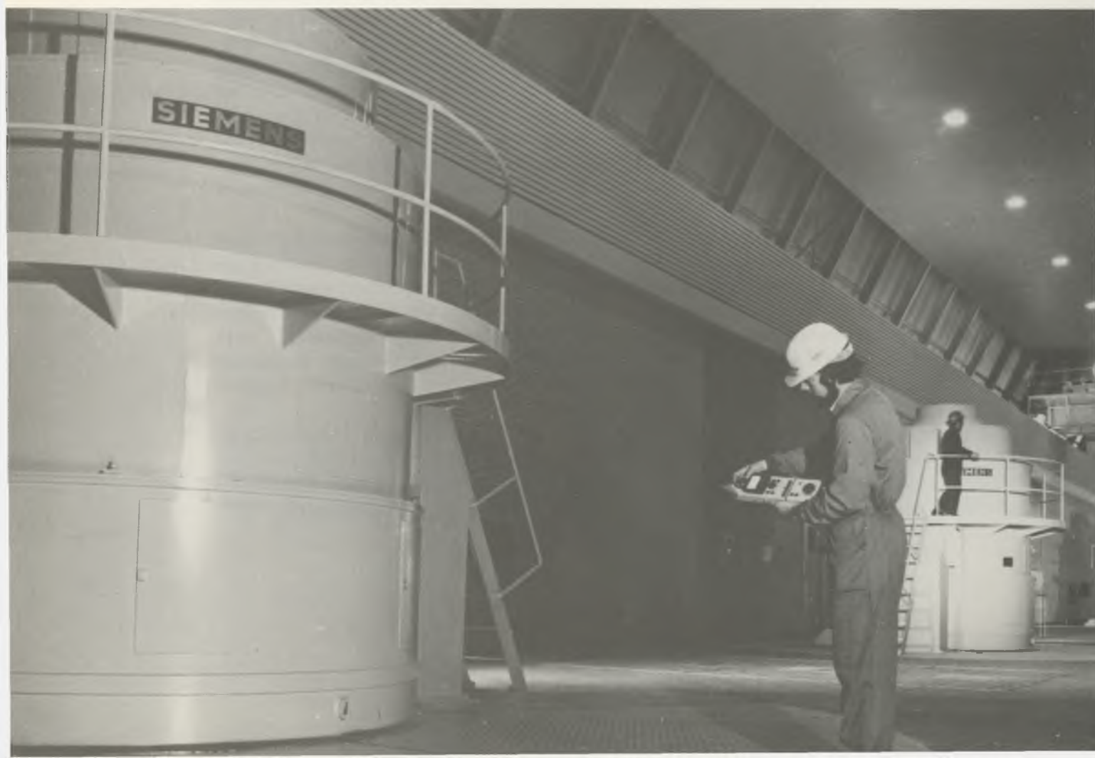
Generator hall, Turlough Hill Power Station.
